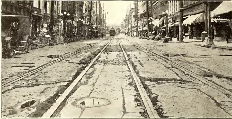
ELMIRA TRACK RECONSTRUCTION — FIG. 1 — CONDITION OF TRACK AND PAVING BEFORE RECONSTRUCTION
